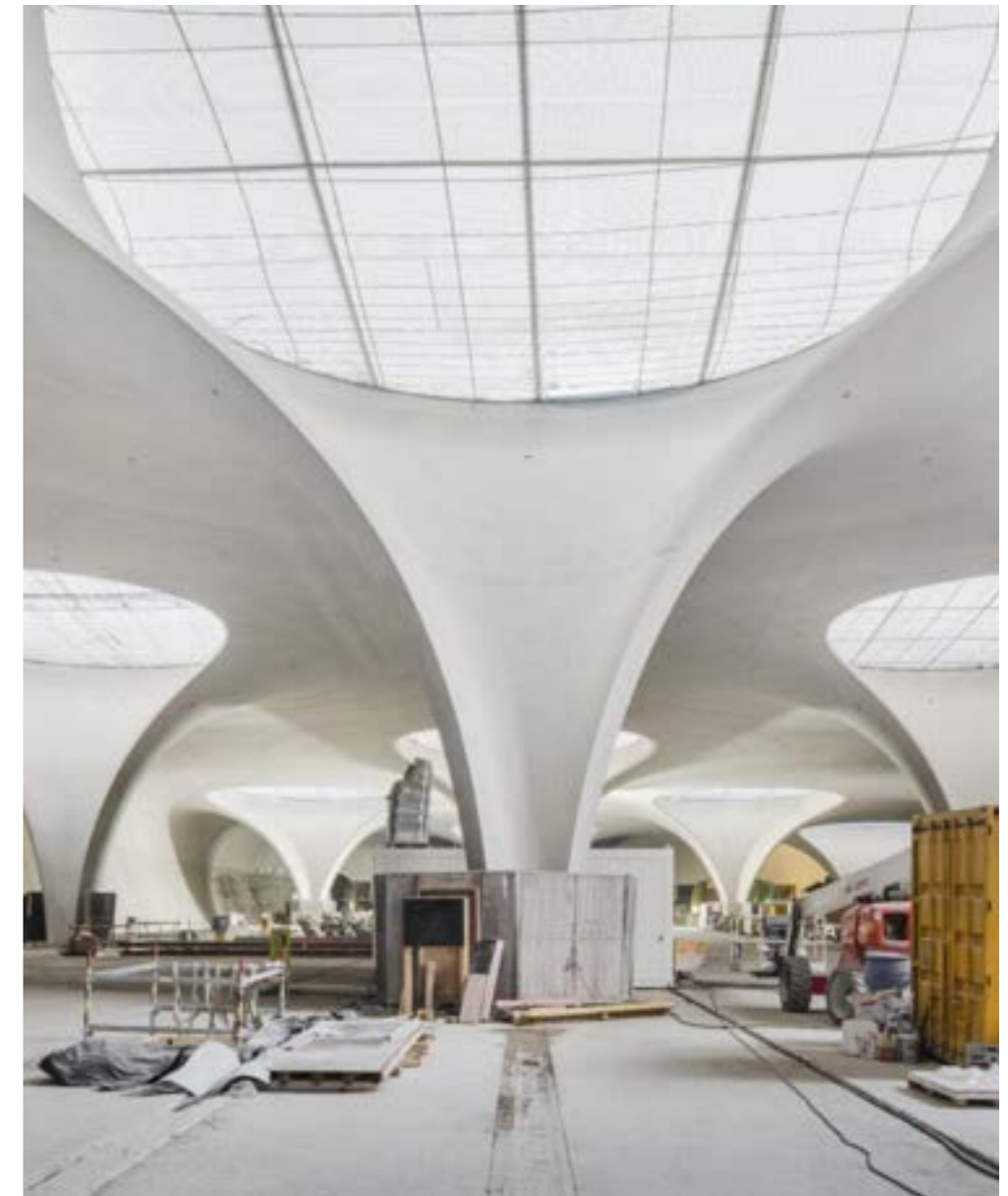
Referentie treinstation Stuttgart - daglichttoetreding
