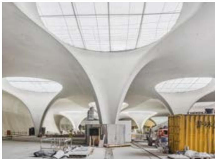
Referentie treinstation Stuttgart - daglichttoetreding
